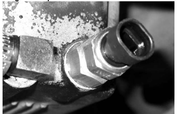
Temp sensor installed as drain plug EVO
